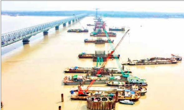
Panoramic Progress: Construction of the Thanlyin Bridge 3 over the Bago River unveiled.
